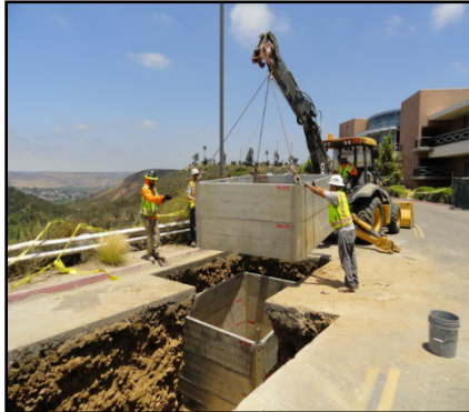
A crew works on the 12kV main service replacement at Grossmont College.
