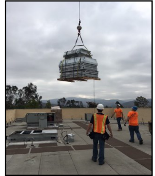
A new HVAC unit is now in place atop the L Building at Cuyamaca College.
